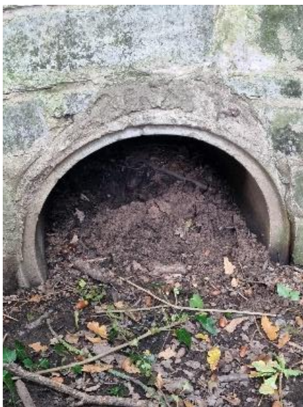
Blocked culverts and drainage have required sustained Council attention.
